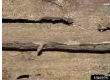
Termite damage (Gary Alpert/IPM Images)
