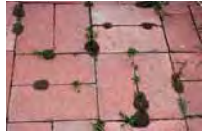
Pavement ant mounds in pavement seams
